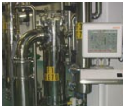
The new automation system
